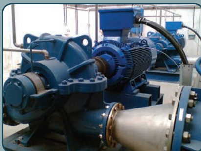
PRAŽSKÉ VODOVODY A KANALIZACE a.s., MAIN PUMPS OF THE PUMPING STATION LIBEŇ, PUMP UNITS CDS SERIES WITH 315 KW MOTORS
