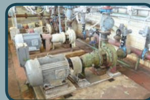
UNIPETROL RPA s.r.o., WASTE MANAGEMENT, PUMPS CSX SERIES IN OPERATION SINCE 1972
