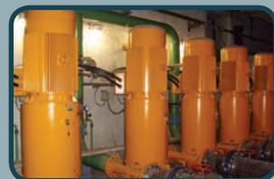
TŘINECKÉ ŽELEŽÁRNY a.s., TERMEX COOLING, UNITS OF THE CSN SERIES WITH 200 kW MOTORS CONTROLLED THROUGH FREQUENCY CONVERTERS
