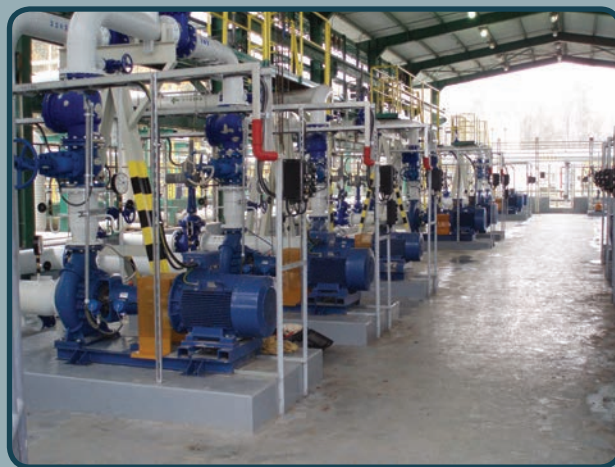
ČEPRO a.s., MAIN PUMPING STATION ROUDNICE – GASOLINE, DIESEL OIL, PUMPS CSI SERIES
