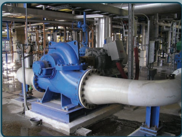
UNIPETROL RPA s.r.o., COOLING CIRCUIT, PUMP UNIT, CDS SERIES WITH THE 315 kW MOTOR, EX CONFIGURATION
