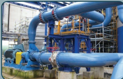
GPN S.A. [FRANCE], PRODUCTION OF NITRIC ACID, PUMP UNIT CSO SERIES WITH 500 KW, 5500 V MOTOR
