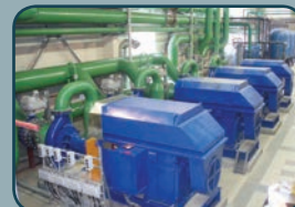
IŽORSKÉ ZÁVODY [RUSSIA], COOLING CIRCUITS, UNITS CSE SERIES WITH 315 KW 6000V MOTORS
