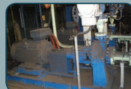
VÍTKOVICE a.s., PRESSURE BOOSTING IN PROCESS TO 80 BAR, PUMP UNITS CSA SERIES, STORAGE OH2
